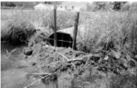
Figure 1. Plugged culvert pipe. Beavers typically use mud, sticks, and other debris to plug culverts. Culvert plugging activity is usually highest during the spring and fall.
