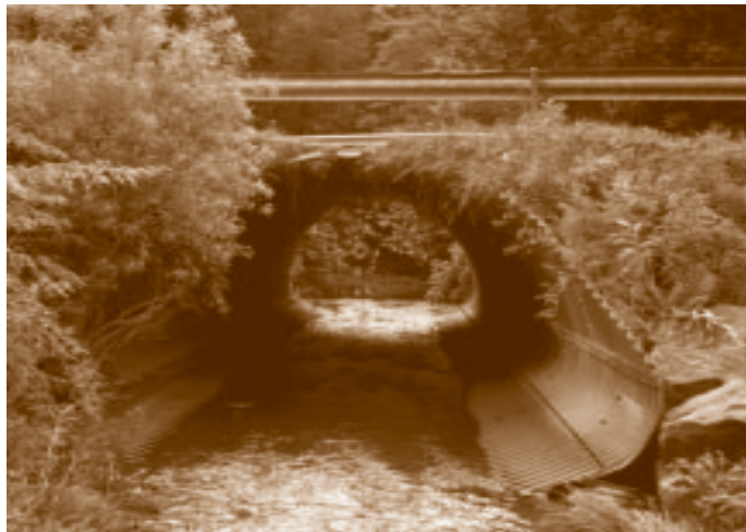
Figure 4. A pipe-arch culvert. These structures may be less prone than round culverts to being plugged by beavers, most likely because they maintain the natural stream width. Additionally, pipe-arch culverts are generally large culverts.
