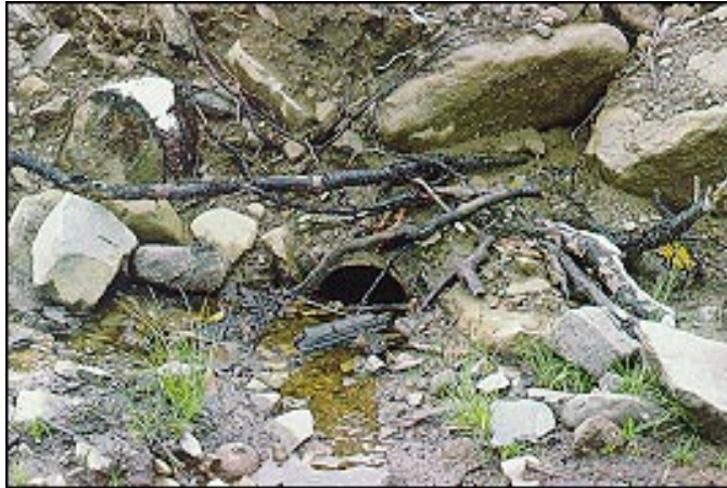
Undersized culverts can become plugged with sediment
