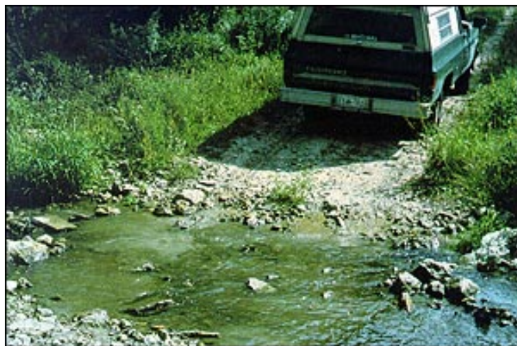
Fords can be an economical method of crossing streams under certain low water conditions and when properly located and designed.
