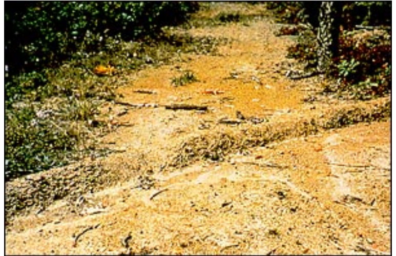
A water bar effectively intercepts surface water and diverts it from the road.
