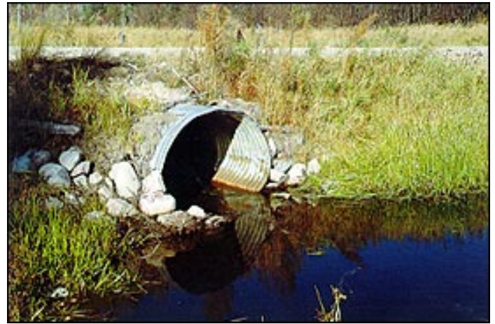
Culverts not installed at the same level as the stream cause water to back up.
