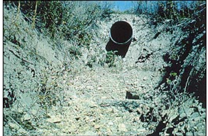
A culvert not installed at the existing stream gradient can degrade the stream channel.
